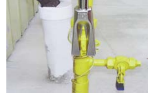
4. Gas Line Shut Off
